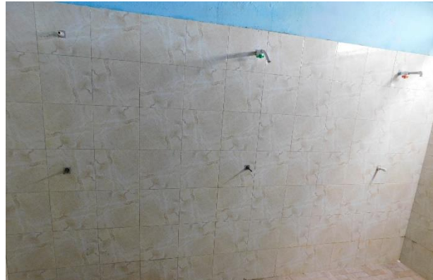
Image 4: Shower with broken fixtures
